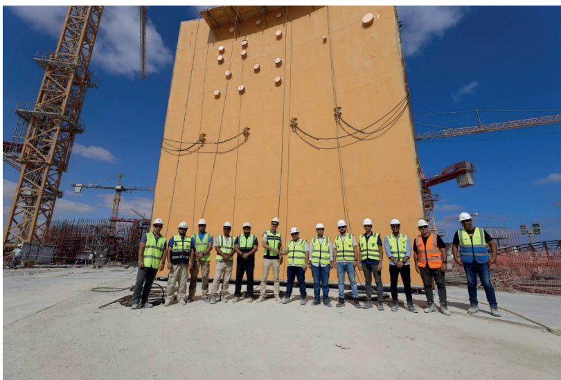
Construction workers at Unit 2, of the El Dabaa Nuclear Power Plant in Egypt.
